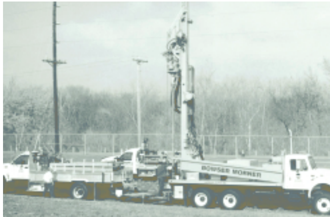
Setting up the sonic rig at a job site in Cincinnati, Ohio.
